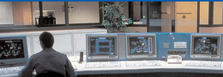
In the control room of Dombasle plant
